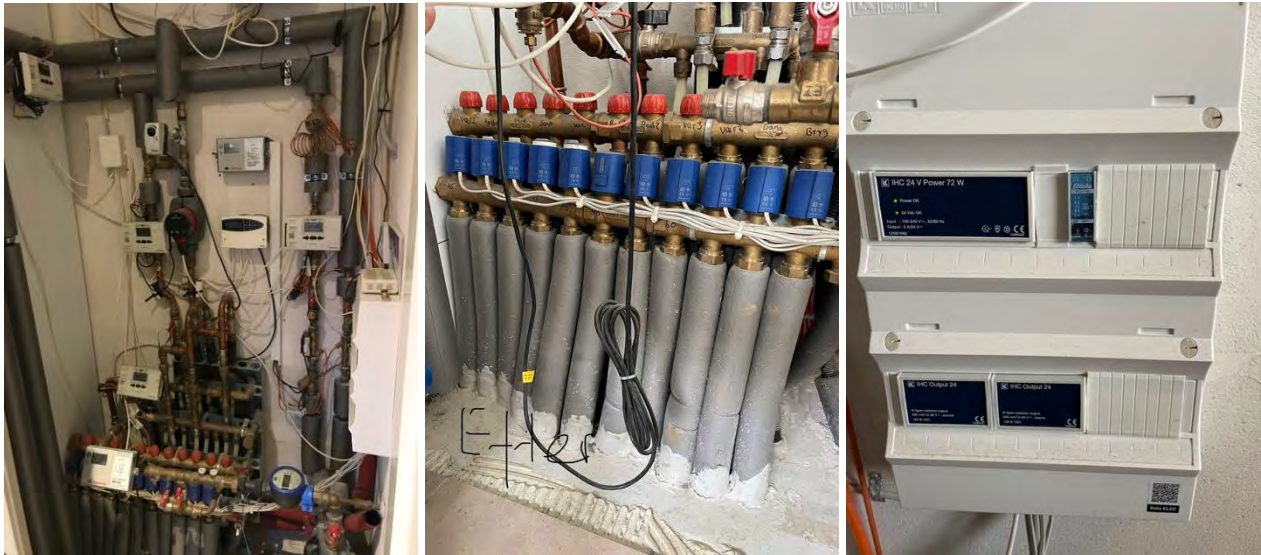
Figure 10: The heating system, from left to right: Technical room with heating installation, the DH enters in the lower right corner, the ECL Comfort 110 and pump in the middle, and the UFH manifold in the bottom. Manifold with Wavin actuators. IHC modules to control actuators.
