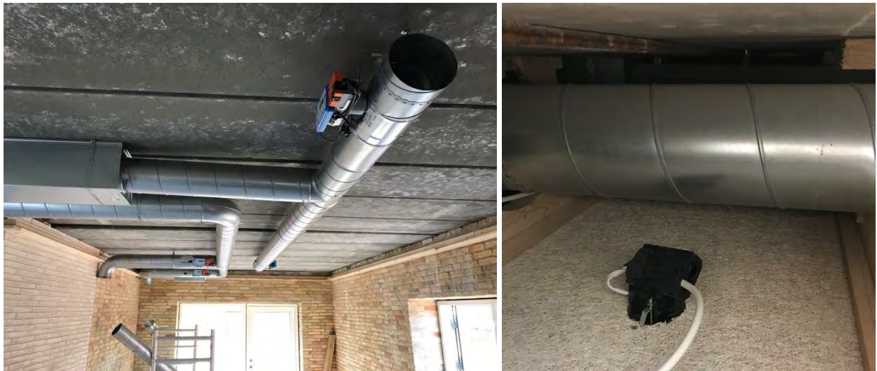
Figure 66: Left picture: Ducts and dampers for supply and extract in the kitchen before the suspended ceiling is installed. Right picture: Duct above the suspended ceiling.
