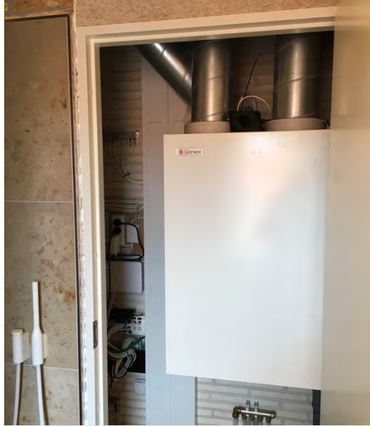
Figure 65: The AHU, Genvex ECO 375TS ALU, located in the technical room on the 1 st floor.
