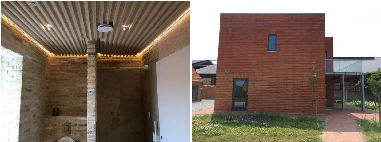
Figure 67: Left picture: Extract diffuser mounted in the ceiling panels in the bathroom on the 1 st floor. Right picture: Exhaust diffusers on the east facade of the building.
