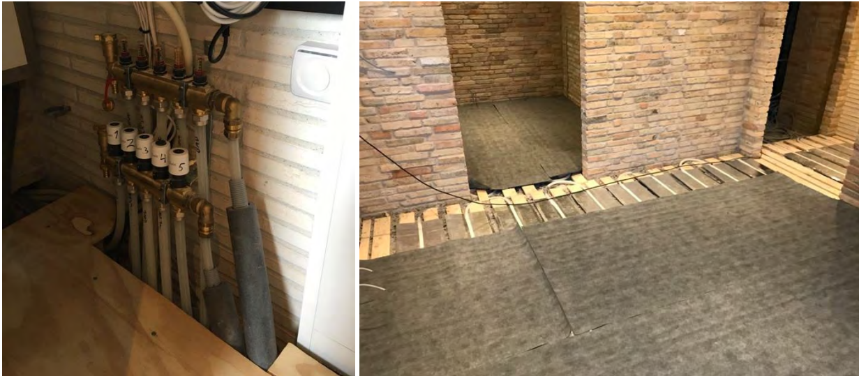
Figure 69: Left picture: Manifold and actuator to the UFH on the 1 st floor. Right picture: The light UFH on the 1 st floor.
