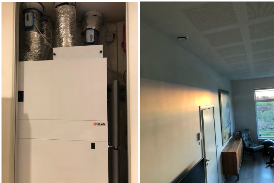
Figure 8: Left picture: The AHU Nilan Compact P with two Lindab UltraLink FTMUs placed on the supply and exhaust main ducts. Right picture: Supply diffuser in the ceiling in the living room.
