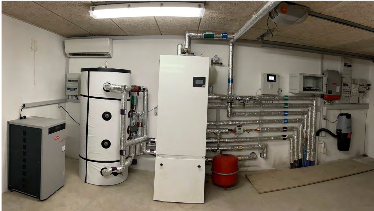
Figure 74: Technical installation in the garage. From left to right: PV battery, heat storage tank, cabinet with ground source heat pump and buffer tank, pipes to the building (DCW, DHW, UFH), pipes to the ground source brine, pipes to the air-to-water heat pump, PV inverter, and electrical board for the installations in the garage.
