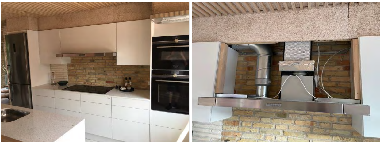
Figure 68: Left picture: In the kitchen a cooker hood is placed above the stove and a cooker hood above the ovens. Right picture: The cooker hood above the stove is a rebuilt model. The standard exhaust part is to the left, and the extension part is the HEPA filter to the right. The extension part recirculates the air after the HEPA filter.
