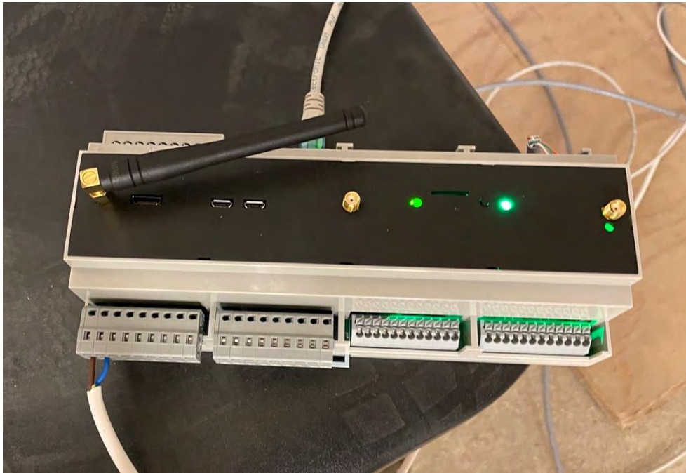
Figure 79: Neogrid's Avenger box - a gateway between Preheat and devices in the building.
