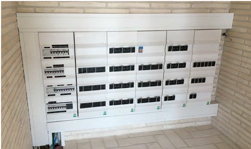
Figure 78: The main switchboard in the house. The first row to the left is normal electrical safety devices. The rest is Niko Home Control.
