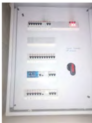
Figure 7 Floor electric panel
