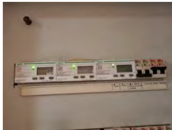
Figure 11 BMS floor meters
