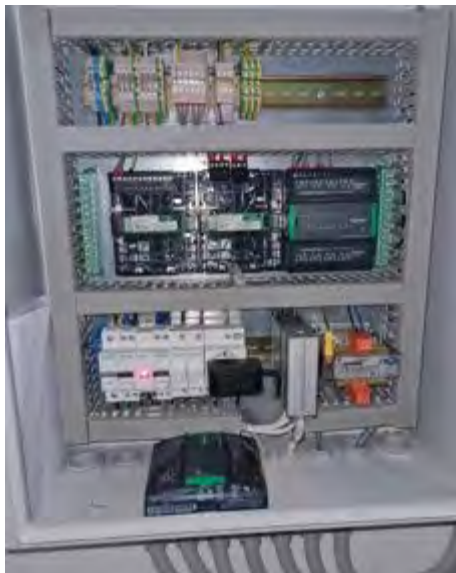
Figure 12 BMS installation general panel
