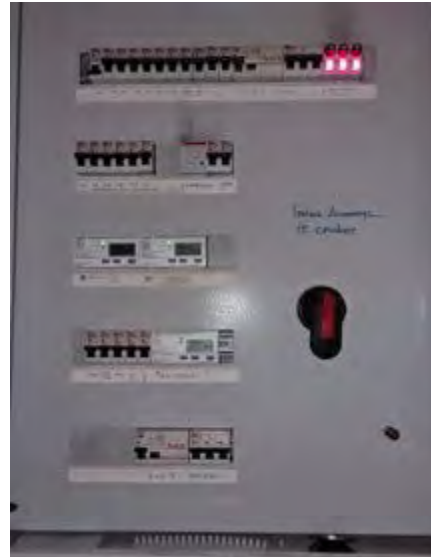
Figure 9 General electric panel
