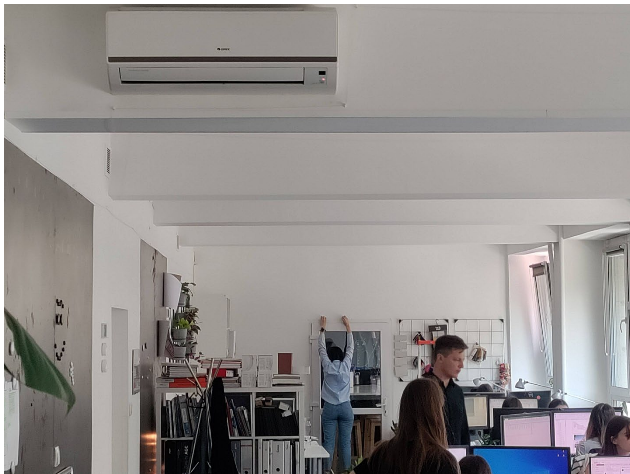
Figure 21. General view of the office with the fiber installed
