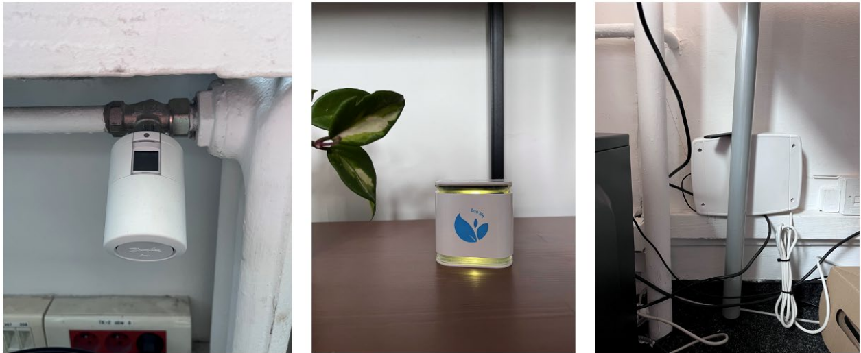
Figure 16 Photographs of installed devices
