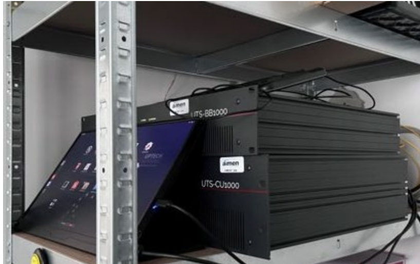
Figure 23. Distributed interrogator installed in BLOK.
