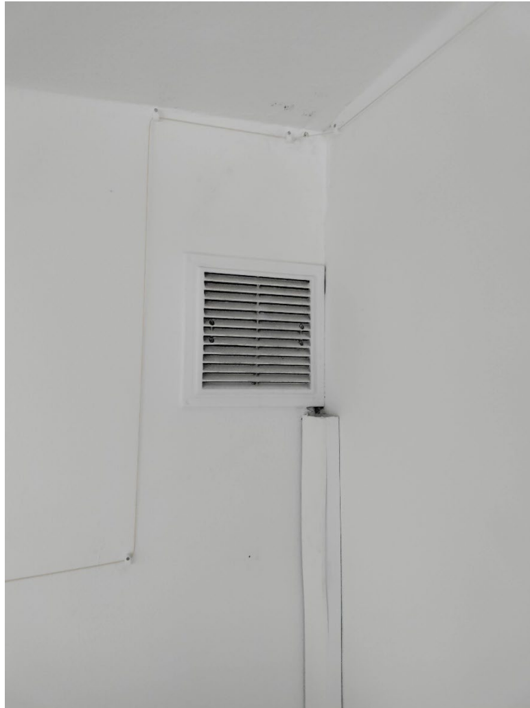
Figure 22. Detail of the fiber installed in a corner of the office
