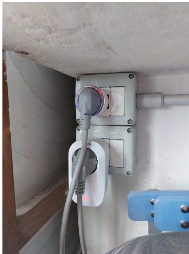
Figure 7 Smart plugs installed in the demo site apartments
